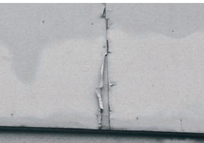
Coatings will not remain adhered if water is permitted to absorb into the material it is intended to protect and is possibly peeling as shown in the above photo.
