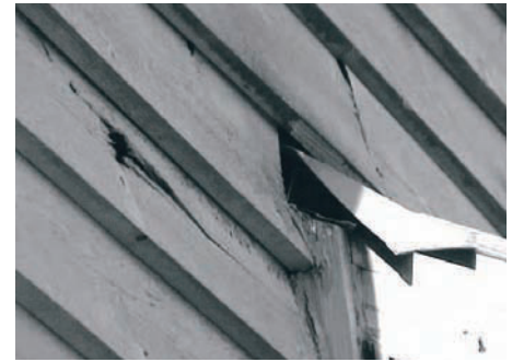
This wood siding has suffered irreparable, permanent damage that cannot be corrected by further paint or stain application. This could have been prevented through proper maintenance.
