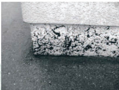
Some coatings such as this acrylic stucco coating over tar-based damp-proofing are incompatible, resulting in a cosmetic detracting instead of providing protection.
